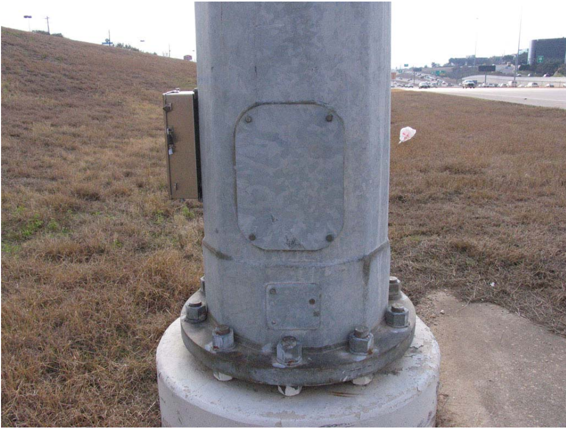
Figure 1.8: Hand access hole for winch system
